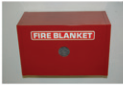
Figure 3-19 Fire blanket storage box. © McGraw-Hill
