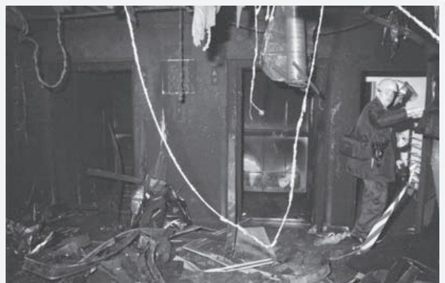
Figure CS12-2 The elevator that brought seven people to the ground floor opened directly into the fire area, trapping and killing them.
