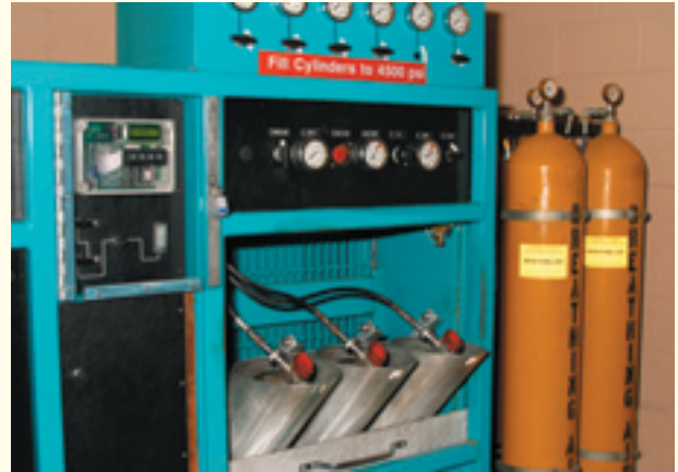
Figure 2-30 Air compressors are installed at many fire stations to refill SCBA cylinders.
