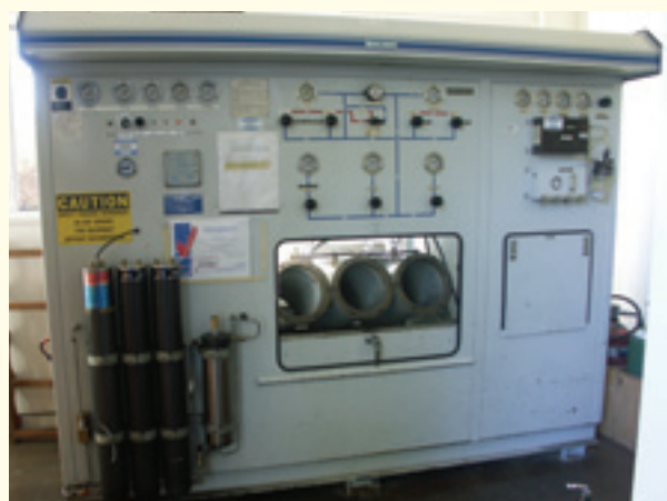
Figure 2-31 SCBA cylinders are refilled in a protective enclosure.
